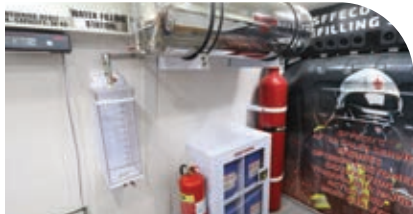
Foam / Water Filling Station
